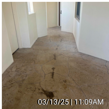
3rd floor stain, spill in walkway. I think I took a picture of this during previous inspec...
