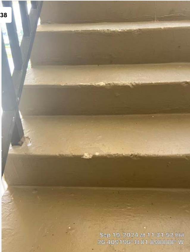
Chipping on stairwell edges, due to long-term wear and tear. Typical of entire stairwell. This is the riser from the 11th floor down to the 10th floor. No action required at this time, although the condition could eventually create a trip hazard and should be monitored periodically.
