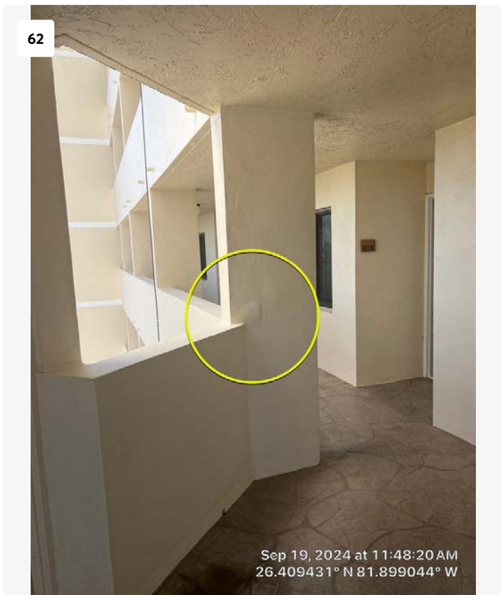
Adjacent to 6th floor elevators. Stucco delamination noted on column--stucco repair is required, and a structural concrete repair may also be needed. Unable to determine until stucco is removed.
