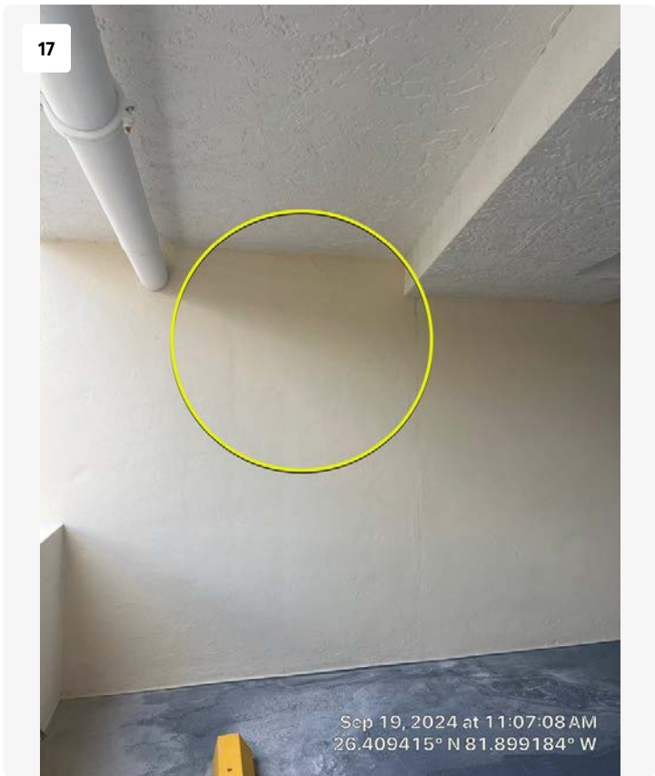
North garage entrance. A crack-like pattern was observed on the wall, although on closer inspection this appears to be a texture mismatch due to a previous repair or removal of paint coatings in the area. No action required.
