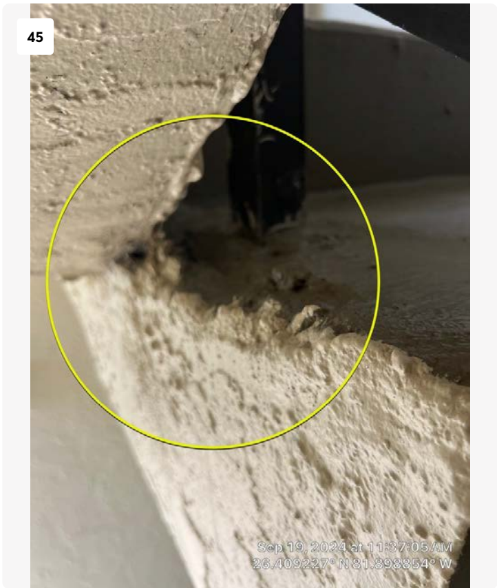
Location of damaged concrete observed on riser headed down to 9th floor. This appears to be related to original construction of the building, likely due to imperfect concrete consolidation. No action is required at this time.
