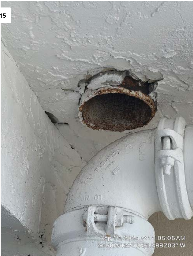
Detail photograph of corroded drain pipe located on northeastern corner of garage.
