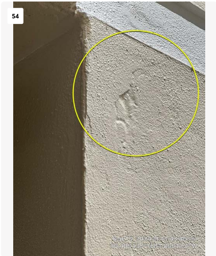
Just to the south of the 7th floor elevators. Previous repair noted. No action required.
