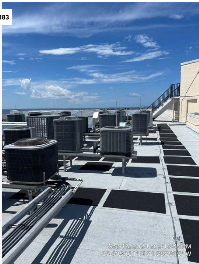
Looking north on roof at Riviera Club. Overall condition of roof appears to be very good.
