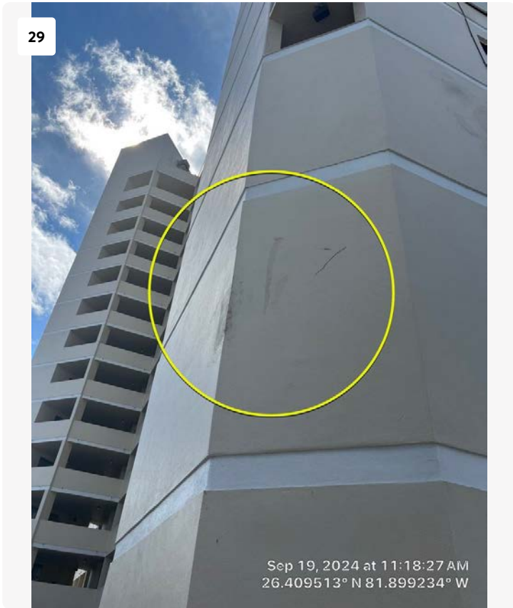
Northeast elevation, corner of building. Texture mismatch and discoloration suggests prior repairs being performed.
