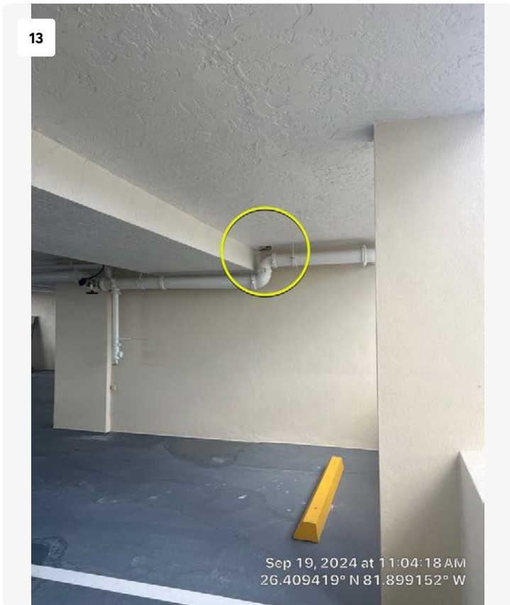
Northwest corner of garage. Corrosion noted on drain pipe.
