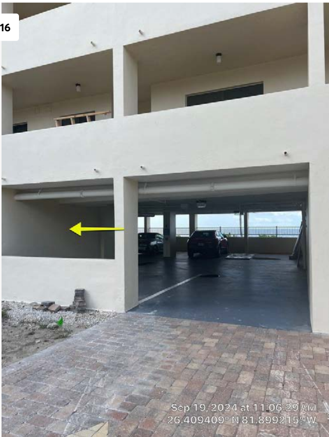
North garage entrance. Coating texture mismatch noted on wall.
