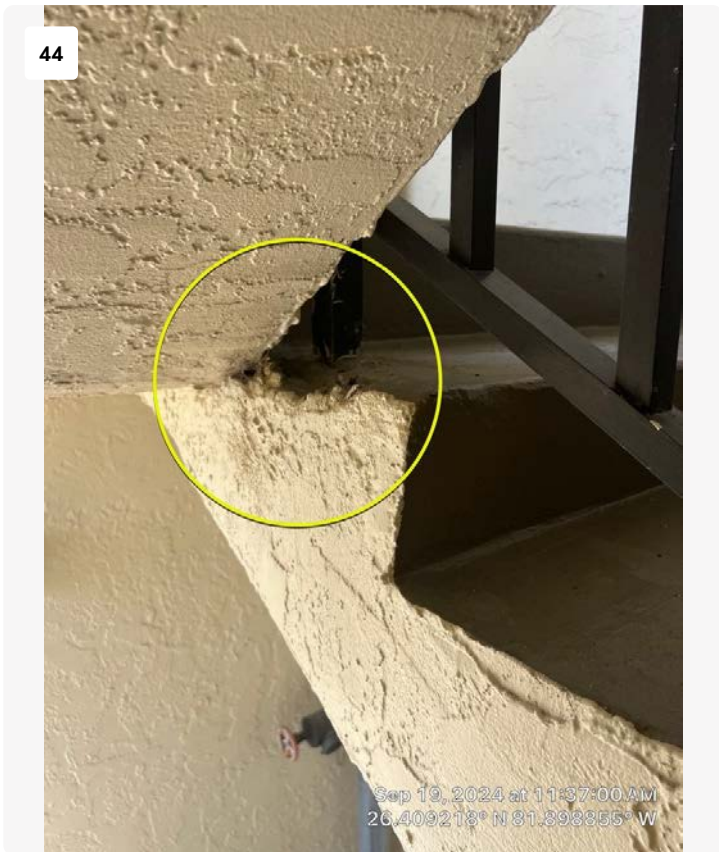
Location of damaged concrete observed on riser headed down to 9th floor. This appears to be related to original construction of the building, likely due to imperfect concrete consolidation. No action is required at this time.
