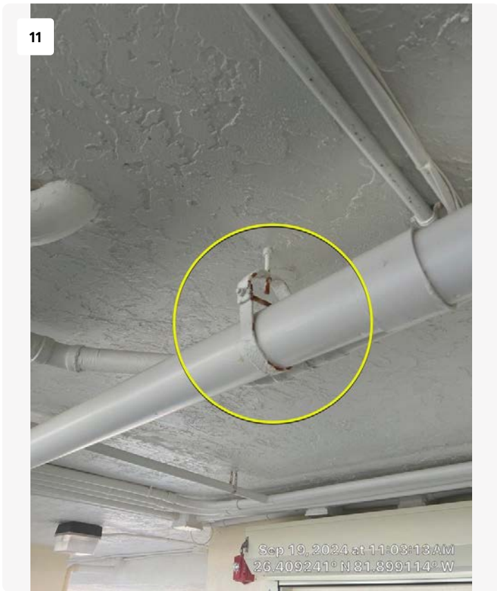
Minor corrosion observed on hangers located just outside garage entrance doors. These areas should be cleaned and repainted, although they will continue to rust and will eventually require replacement.
