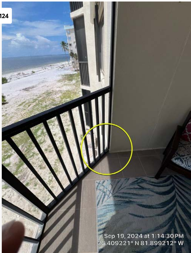
Small crack in slab edge on balcony of Unit 204. This is very likely a concrete spall which needs to be repaired to prevent moisture intrusion into the slab.
