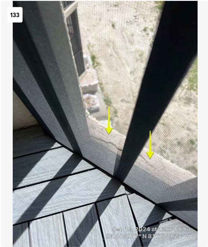
Concrete Spall requiring repair at slab edge of balcony 303.
