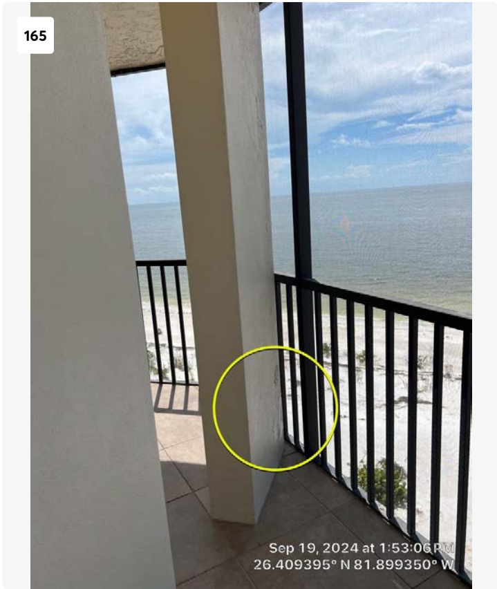
Possible previous repair noted on balcony column Unit 601.
