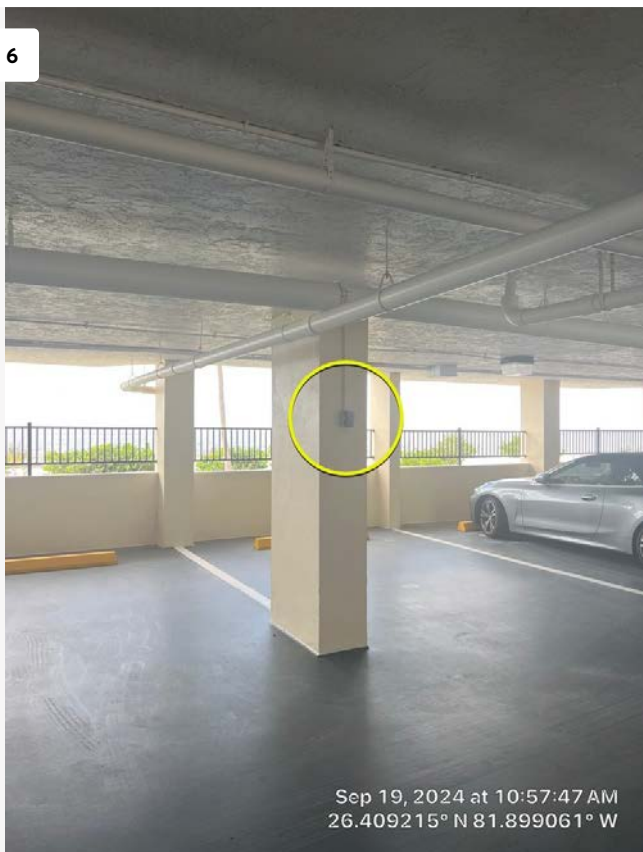
Open electrical junction box in garage just outside of elevator entrance door. This needs to be repaired.
