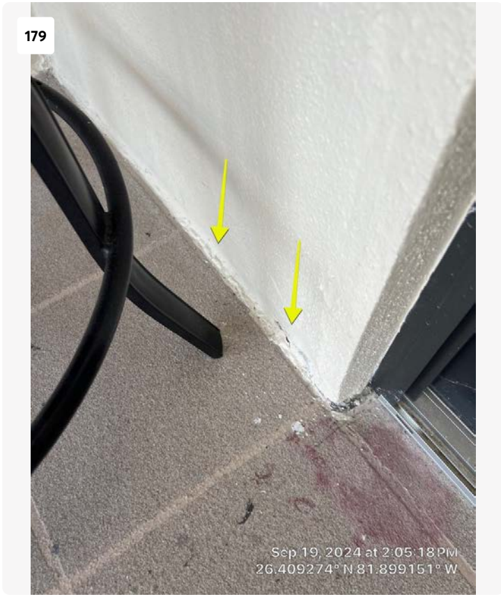
Small crack noted just outside slider on balcony of Unit 804. This area should be repaired to help prevent moisture intrusion into slab.
