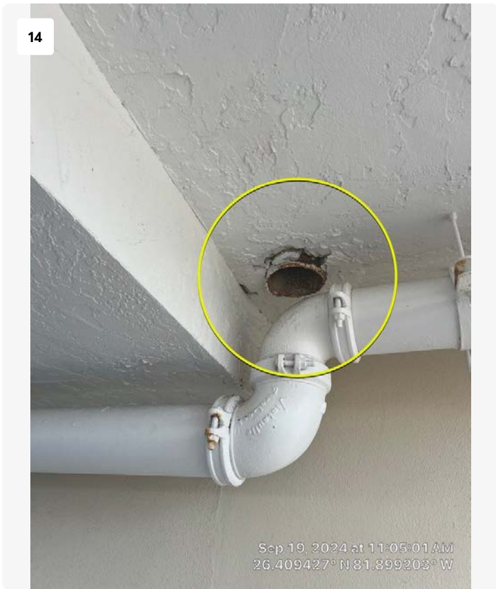
Northwest corner of garage. Corrosion noted on drain pipe. It is unclear if this pipe has been abandoned previously. No immediate action appears to be required, although eventually the pipe will rust and then contribute to concrete spalling in the surrounding slab.
