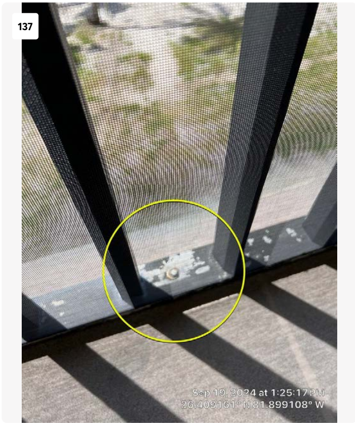
Very minor corrosion observed on guardrail fasteners of balcony Unit 305.
