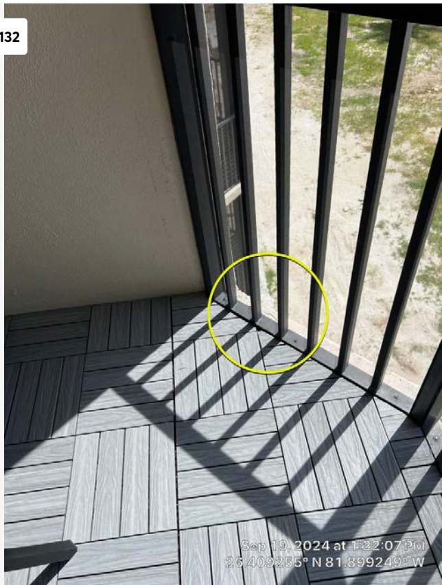
Concrete spall in slab edge of balcony 303. Requires repair.
