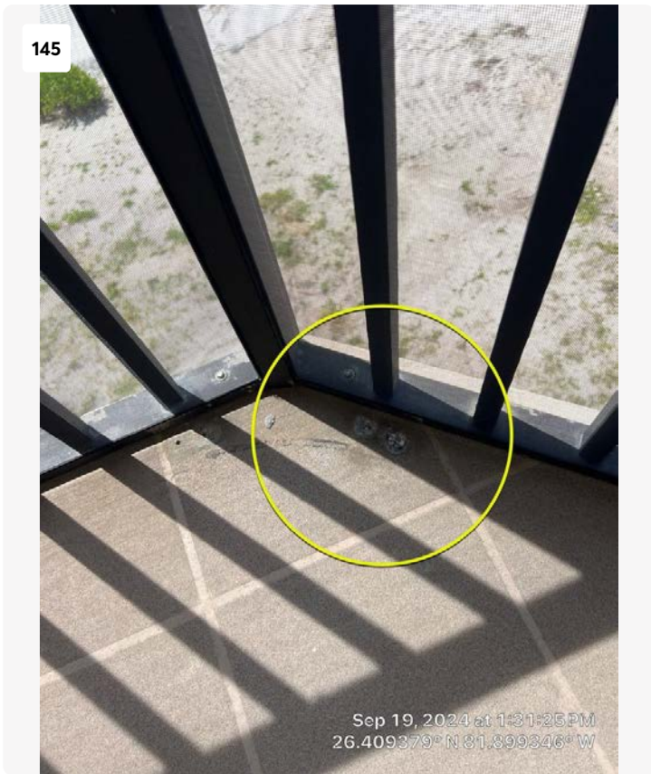
Unrepaired railing attachment points on floor of balcony Unit 401. These locations should be coated to help prevent moisture intrusion into the concrete slab.
