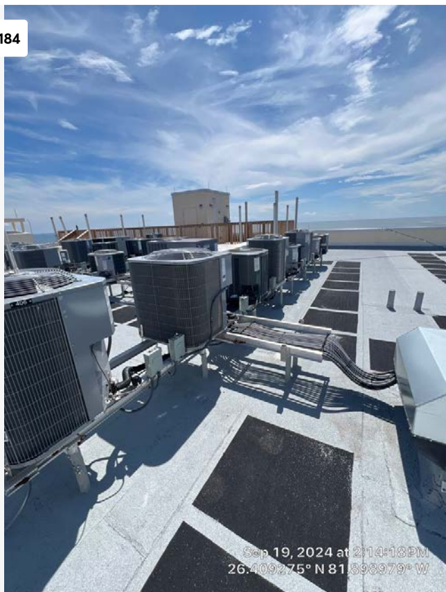
View looking east at AC clusters. All hurricane straps appear to be in like new condition.
