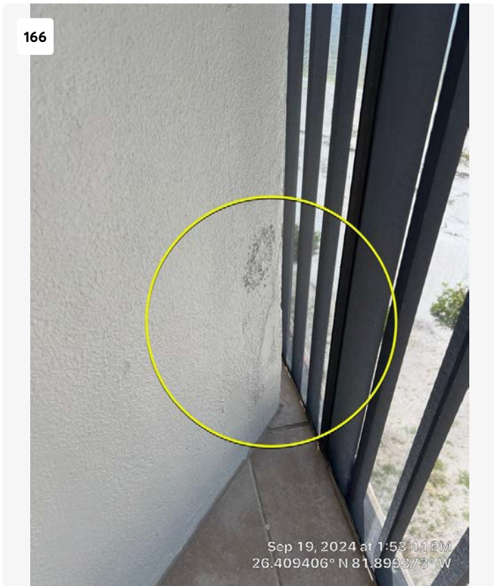
Possible previous repair noted on balcony column Unit 601. No action required at this time.
