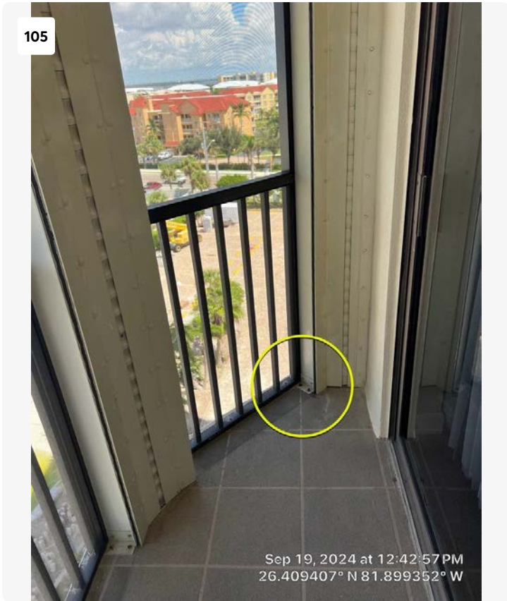
Minor corrosion noted on fasteners on small side balcony of Unit 701.
