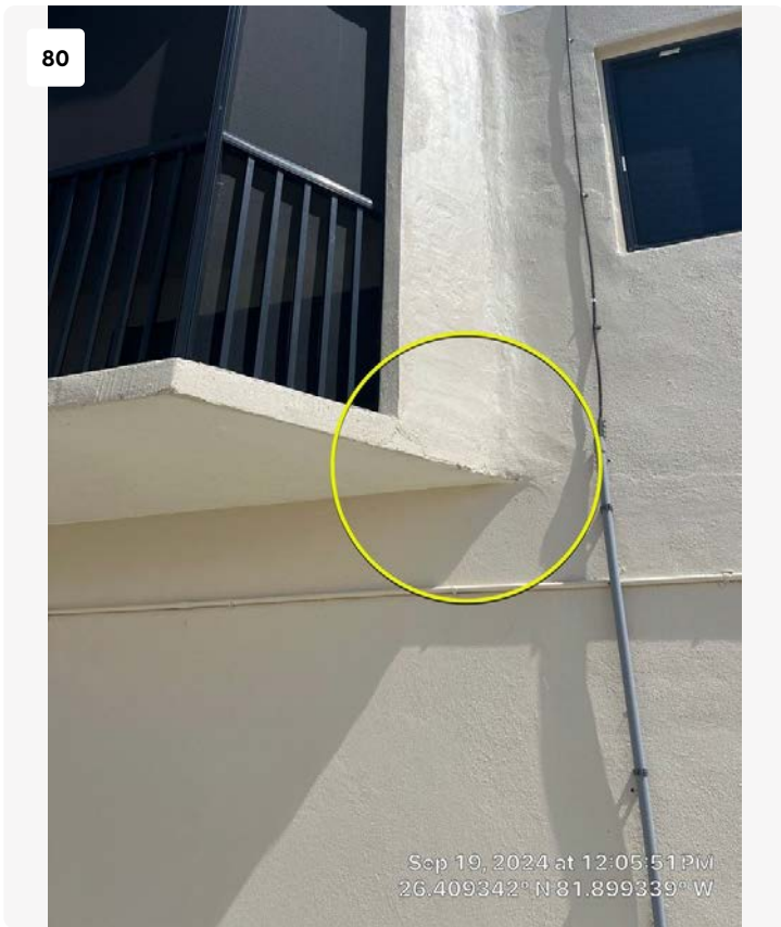
Northwest elevation, first floor balcony. Possible spall observed in balcony slab edge. It may also simply be a prior repair with texture mismatch. No action required at this time.
