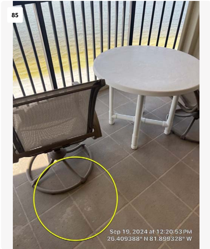
Mild deterioration of balcony coatings observed on balcony of Unit 1001.
