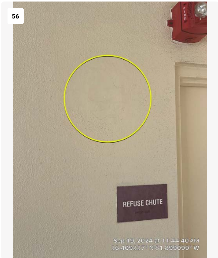
7th floor refuse chute. Previous repair noted.
