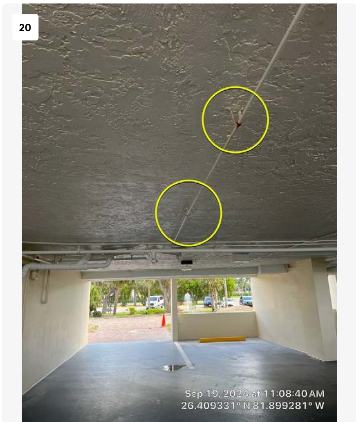
Looking east at north garage entrance. Corrosion noted on hangers. Typical of conditions throughout the garage. They should be cleaned and coated, and may require replacement on an as-needed basis.
