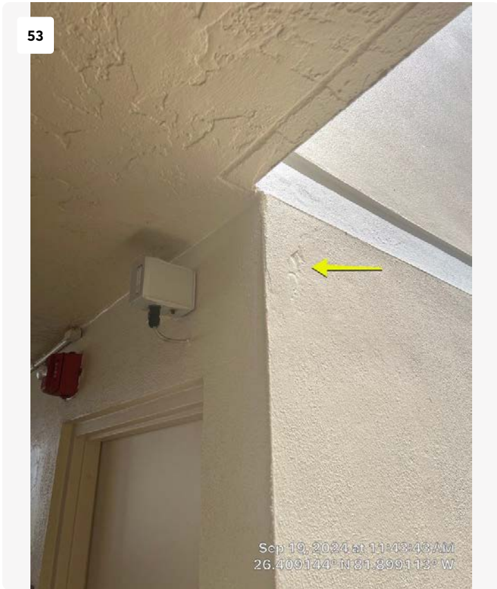
Just to the south of the 7th floor elevators. Previous repair noted.
