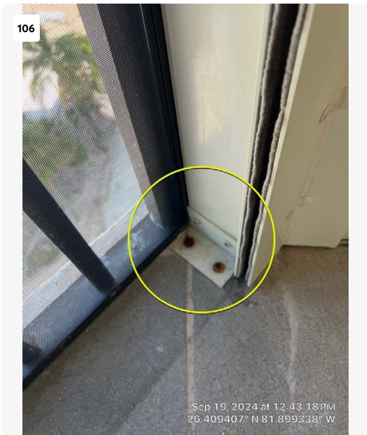
Minor corrosion noted on fasteners on small side balcony of Unit 701. Fasteners like this should be periodically inspected and can be replaced on an as-needed basis.
