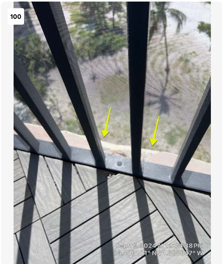
Northwest elevation, first floor balcony. Concrete spall observed at balcony slab edge. This area should be repaired to prevent additional structural deterioration.
