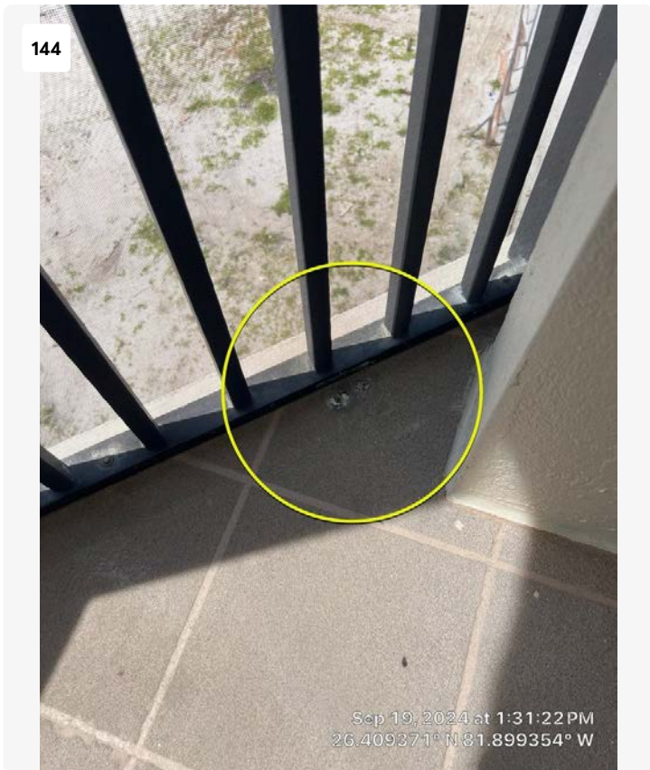
Unrepaired railing attachment points on floor of balcony Unit 401.
