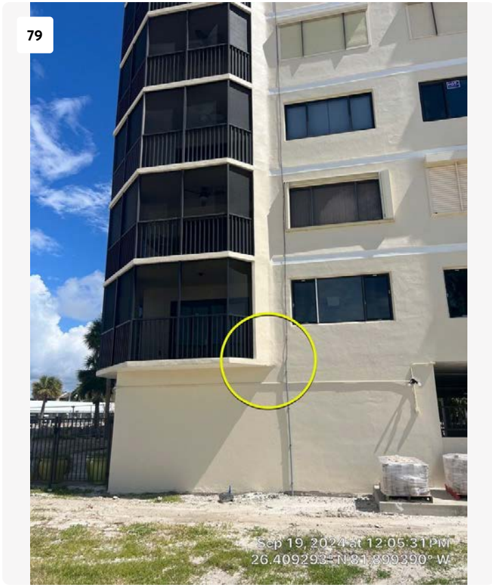
Northwest elevation, first floor balcony. Possible spall observed in balcony slab edge. It may also simply be a prior repair with texture mismatch. No action required at this time.
