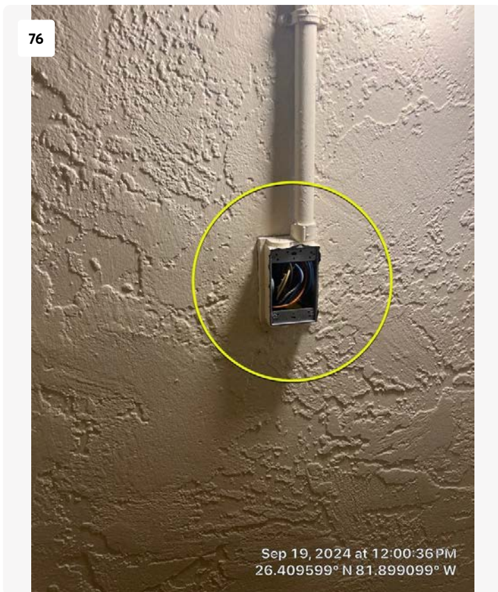
Location of open electrical junction box, 1st floor north stairwell. This box requires repair and a cover plate installed.
