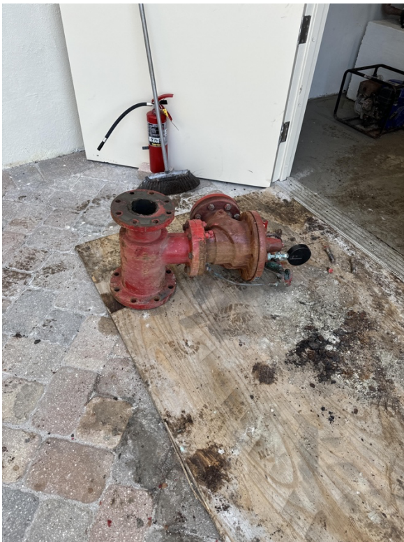
Old Fire Pump Parts
