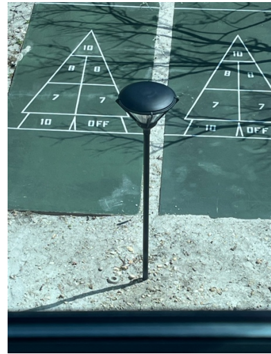
New exterior lights
