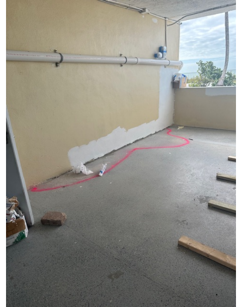
Garage Floor Void
