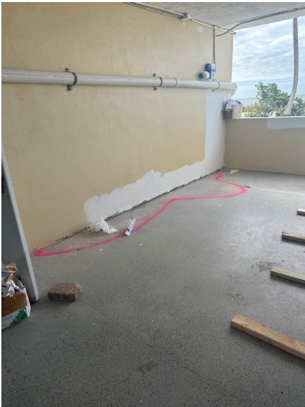
Garage Floor Void
