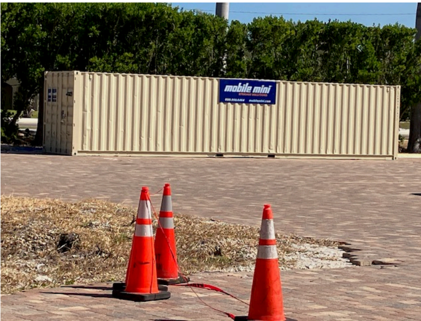
Container with new air conditioning units
