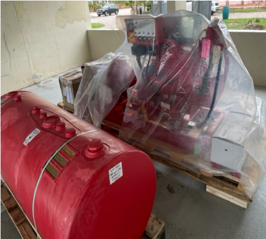
Fire pumps, system.
