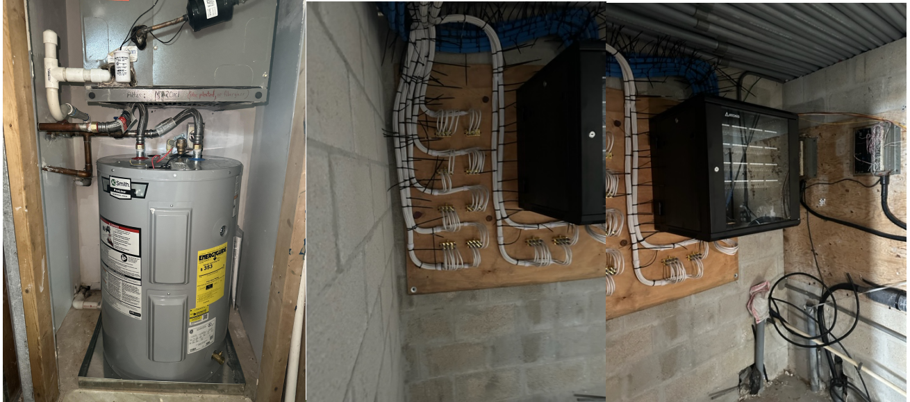
New Hot Water Heater 1 st Floor
