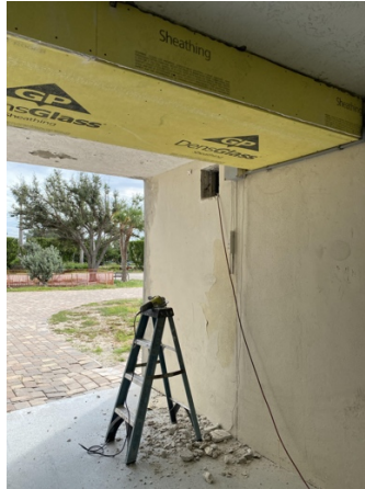
Piping Enclosures in Garage
