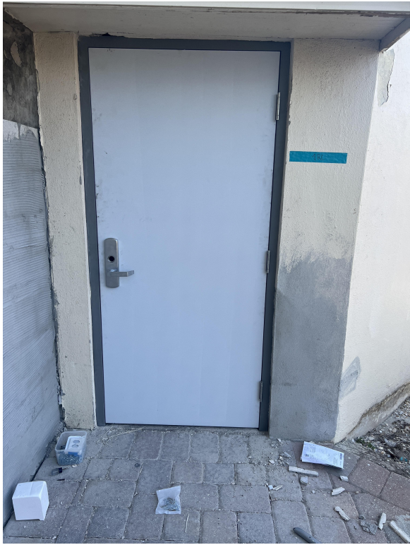
NEW FIRE DOORS INSTALLED
