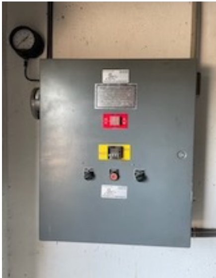
PUMP CONTROL PANEL
