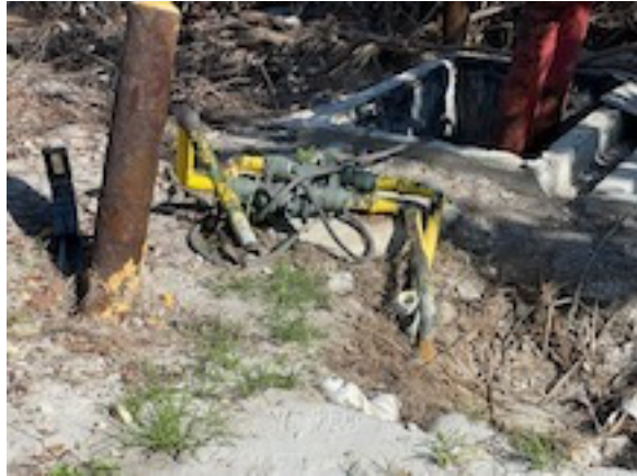
WATER PUMP BACKFLOW SYSTEM
